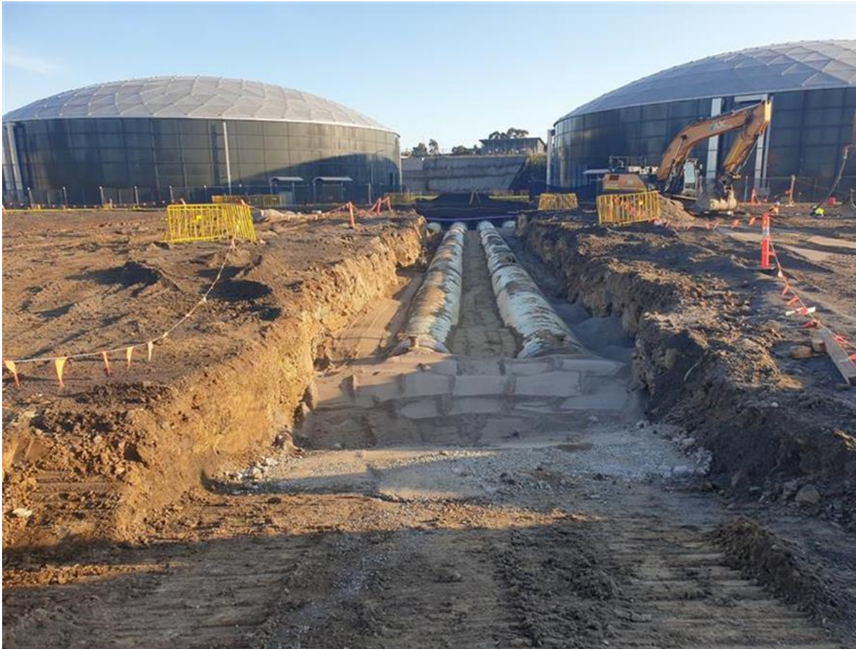
Figure 4: Use of recycled sand as embedment material at a Sewage Flow Control facility
